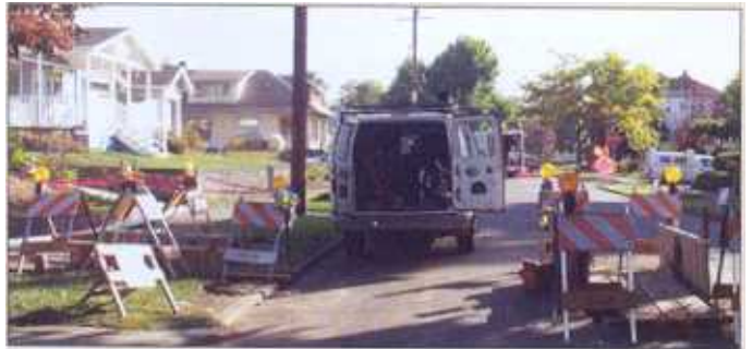
TTC is conducting a study to identify and resolve infiltration and inflow (I&I) issues attributable to sewer laterals.
