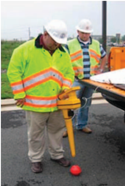
FIGURE 4 A marker ball RFID/Sonde being programmed prior to emplacement. (Photo courtesy of VDOT.)
