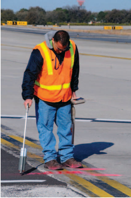
FIGURE 3 EML device in use to designate electric lines. (Photo courtesy of Cardno.)
