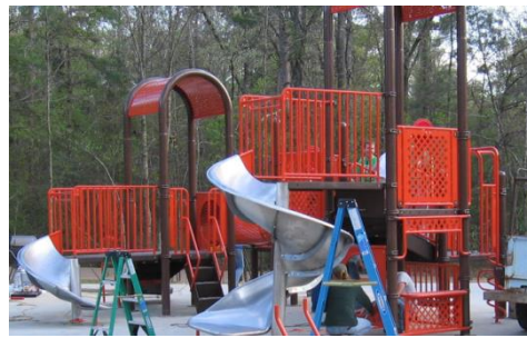
Erected Play System at Cypress Springs with the Engineering and Science Association (2007)
